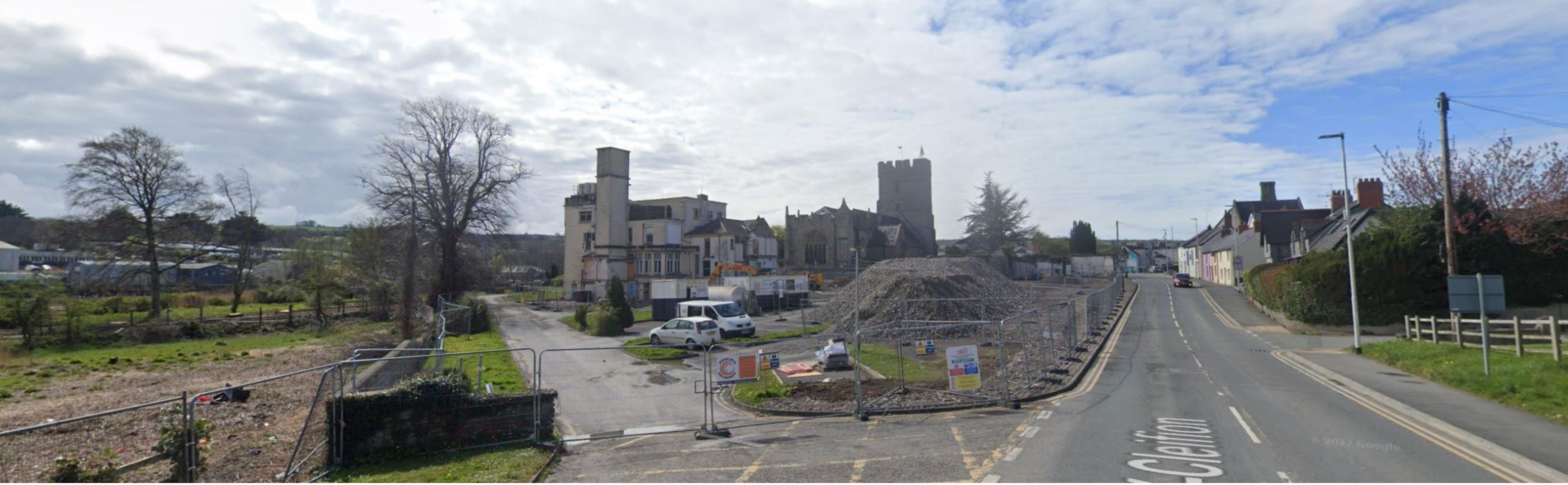
Above: Looking west up Pont-Y-Cleifion with the partially demolished hospital to the left and St Mary's Church behind.
