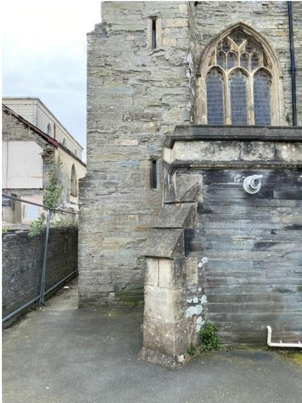
Above: The existing eastern wall of the church, with the partially demolished Memorial Hospital beyond.
