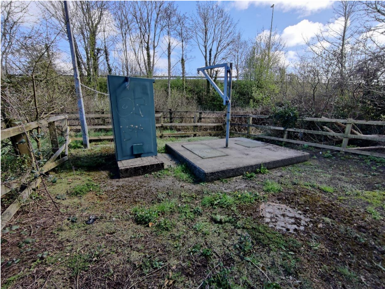
Figure 2-4 DCWW Pumping station.
