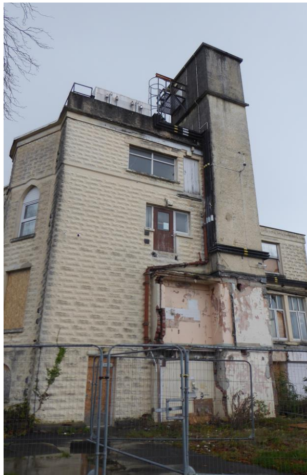
Figure 20 East end as seen November 2023 following demolition of the former single-storey physiotherapy range
