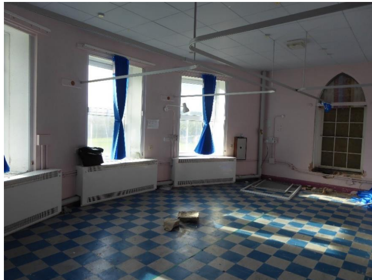
Figure 32 Former Celynnen Ward in ground floor (south and west walls) of Priory House
