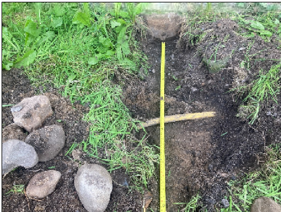
P12: Photograph showing gas main encountered in TP07
