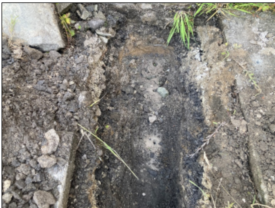
P4: Photograph showing concrete obstruction at base of TP01B
